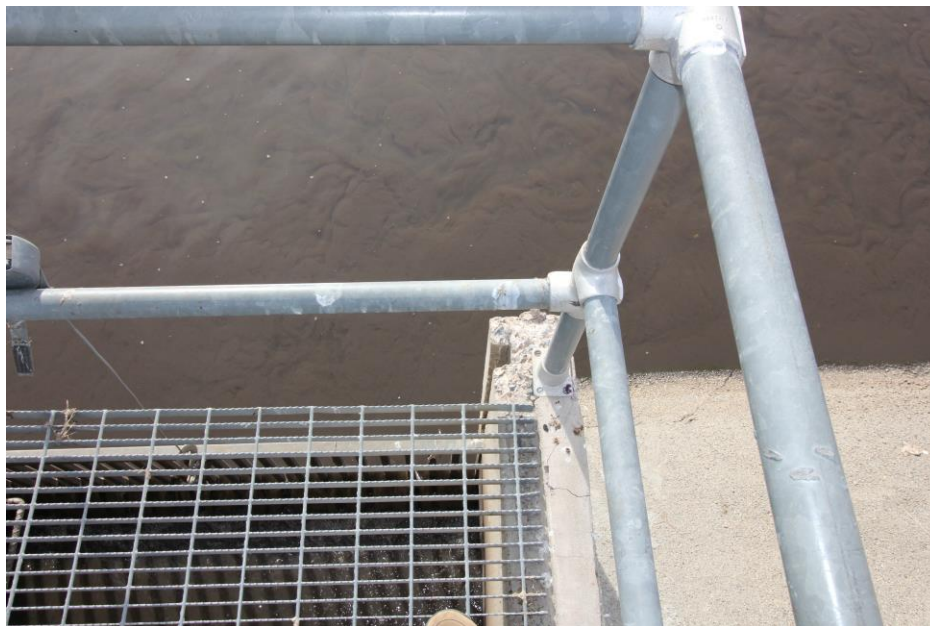
Figure 15: Oxidation Ditch Structural Issues
